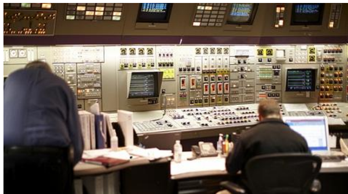
Figure 3-4 Darlington Main Control Room
