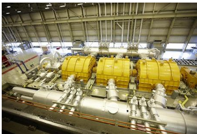
Figure 3-3 Darlington Unit 2 Turbine-Generator
