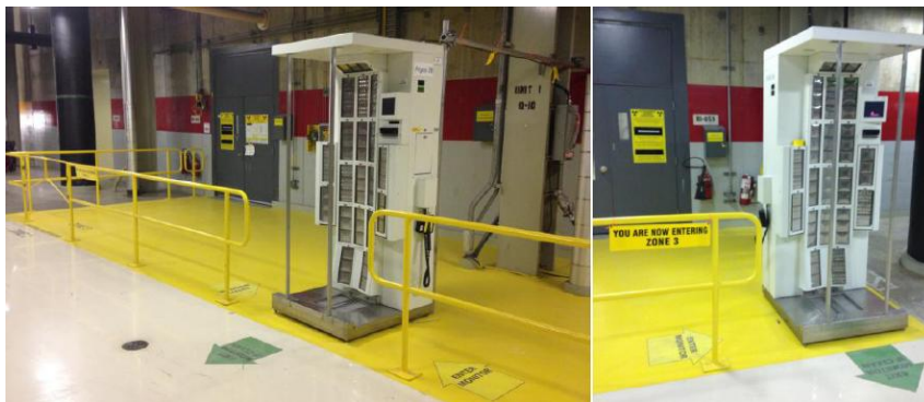
Figure 3-13 Zone Boundary Monitors, Floor Markings and Barriers
