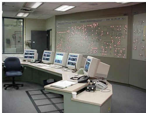
Figure 4-9 TRF Control Room
